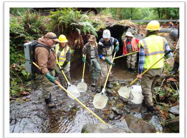
DURING: Prior to any work in the stream channel, partners relocate fish and other aquatic organisms to a safe location outside the work area.
