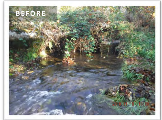
BEFORE: The culvert at Bear Creek was undersized, in very poor condition, and at risk for catastrophic failure.
