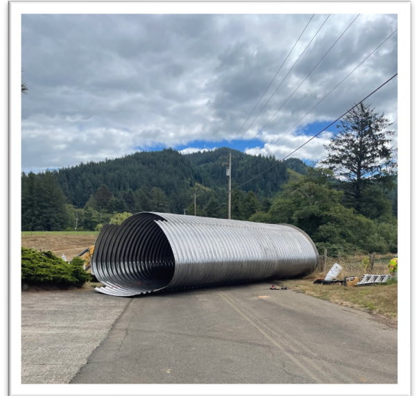
DURING: The arch pipe culvert assembled and ready to be lowered into place.
