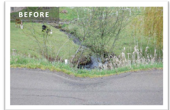
BEFORE: The failing culvert as illustrated by the dip in the pavement directly above it.
