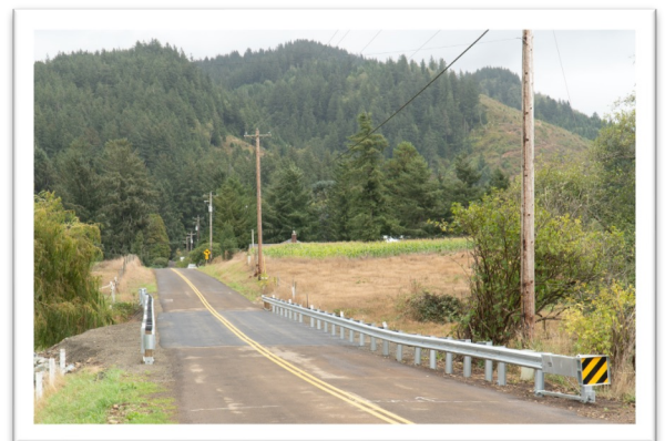
AFTER: The finished project provides local access to landowners along Fairview road and restores access to nearly 2 miles of fish habitat while improving natural stream functions.
