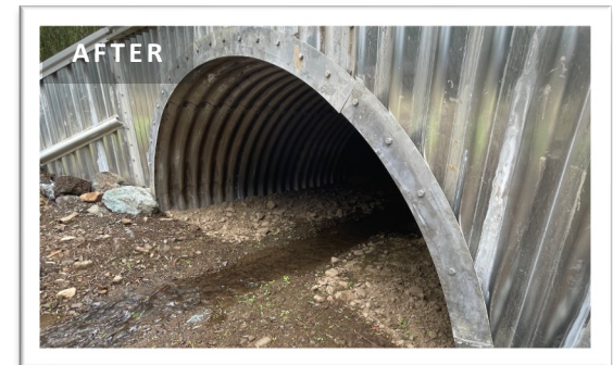
AFTER: The new arch pipe culvert provides ample room for higher flows and restores safe passage for fish under Fairview Road
