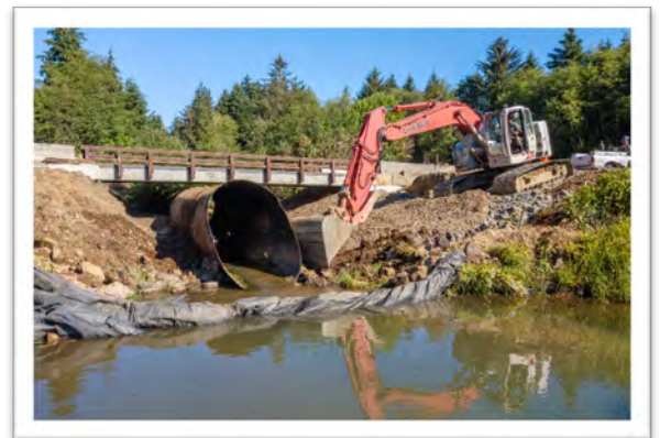
DURING: A temporary bypass bridge keeps traffic moving while the old culvert is replaced with a new bridge.
