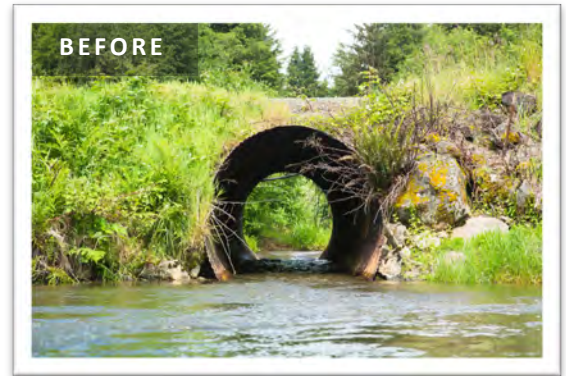
BEFORE: The culvert at Peterson Creek was undersized, in very poor condition, and at risk for catastrophic failure.
