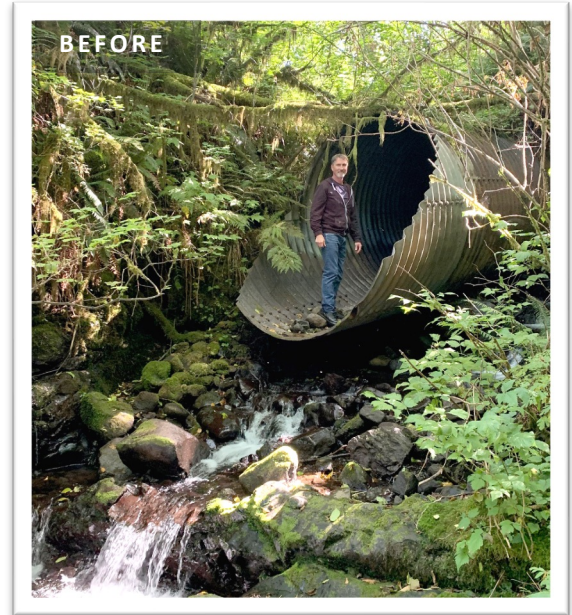
BEFORE: The undersized, perched barrier culvert was so degraded that the stream was running partially underneath the culvert.
