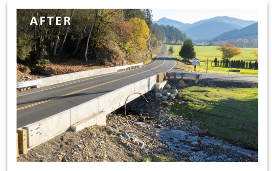
The completed bridge provides safe fish passage and ample room for debris to pass downstream.
