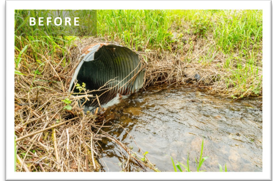
The failing culvert regularly plugged with debris causing flooding.
