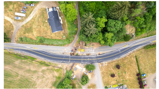
A temporary bypass bridge keeps traffic moving while the old culvert is replaced.
