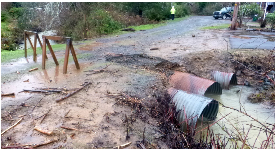
SALMON SUPERHWY PROJECTS REMEDY FLOODING AND FISH PASSAGE FAILURES LIKE THIS ONE.
