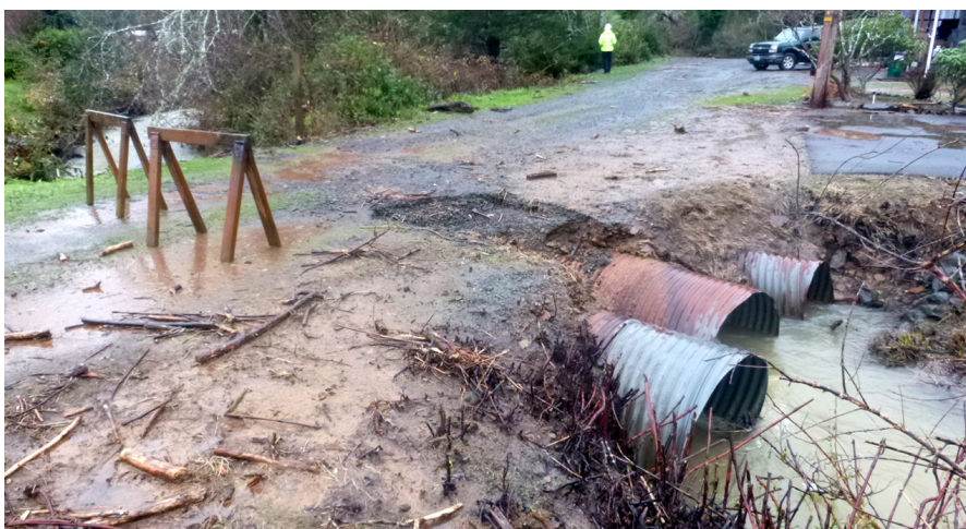
SALMON SUPERHWY PROJECTS REMEDY FLOODING AND FISH PASSAGE FAILURES LIKE THIS ONE.
