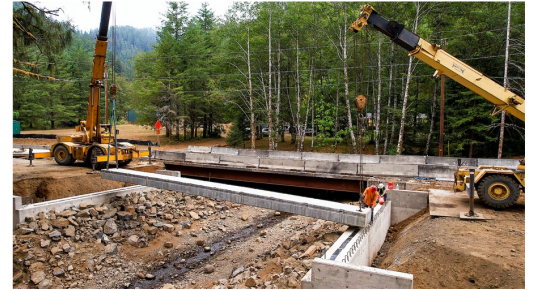
DURING: A temporary bypass bridge keeps traffic moving while the old culvert is replaced.
